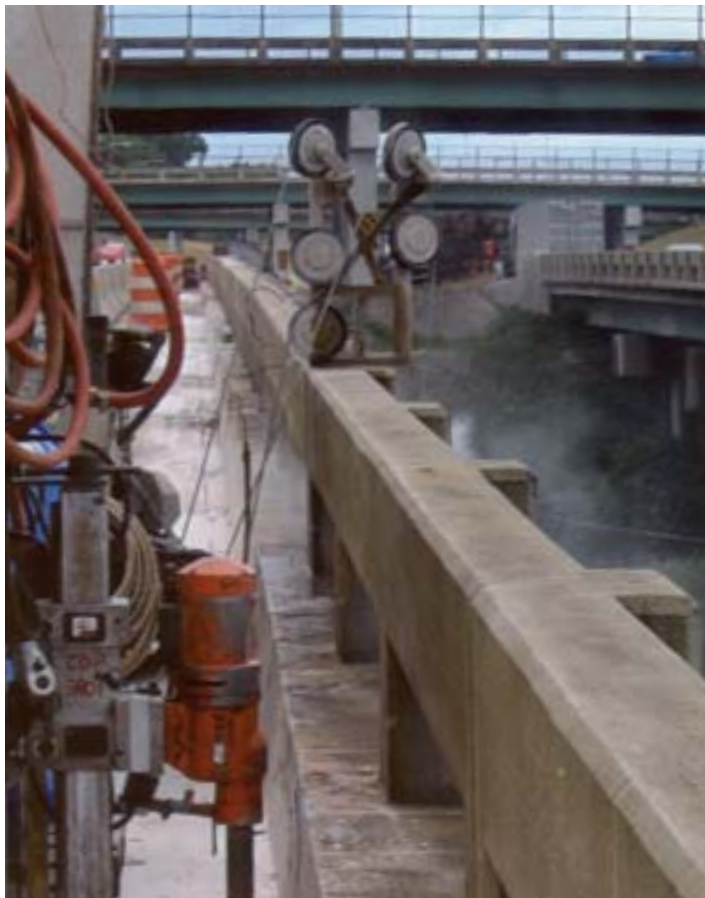
Bridge rails were cut into 50-foot sections to be removed by crane.
